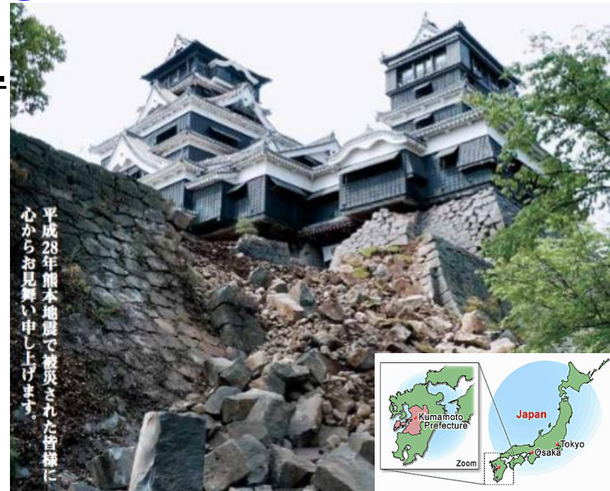
Kumamoto Castle after the Kumamoto earthquake (M6.5+M7.3 Apr.16. 2016)
