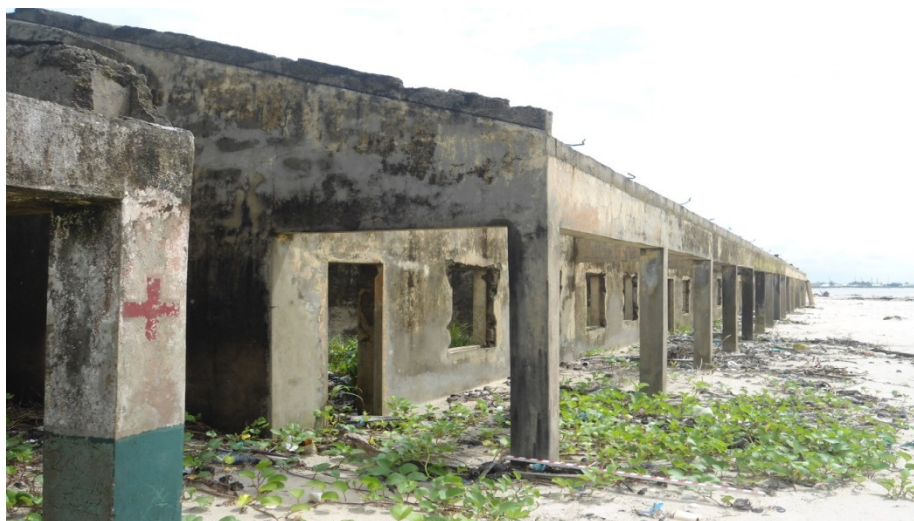
Plate 14: Former Itak Abasi primary School damaged by storm surge in 2011
