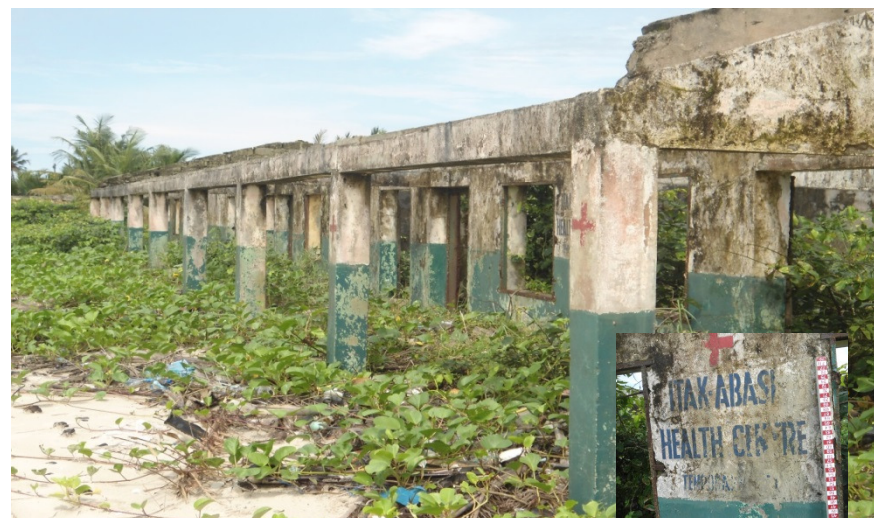
Plate 15: Former Itak Abasi Health Centre damaged by storm surge in 2011
