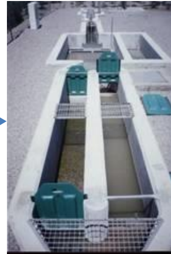
Static grit chamber
