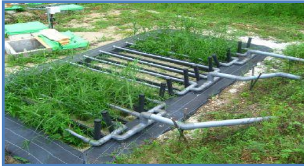
Urban-Industrial wastewater treatment
