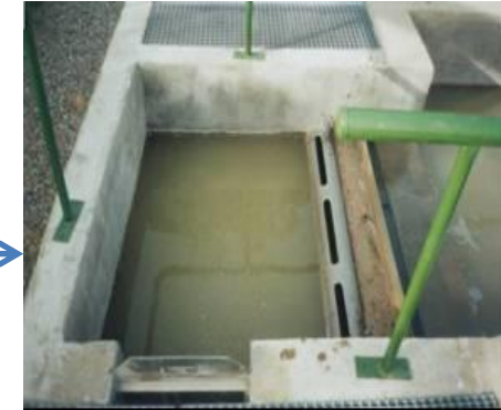
Static grease chamber
