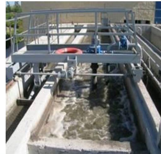
Aerated grit-grease chamber
