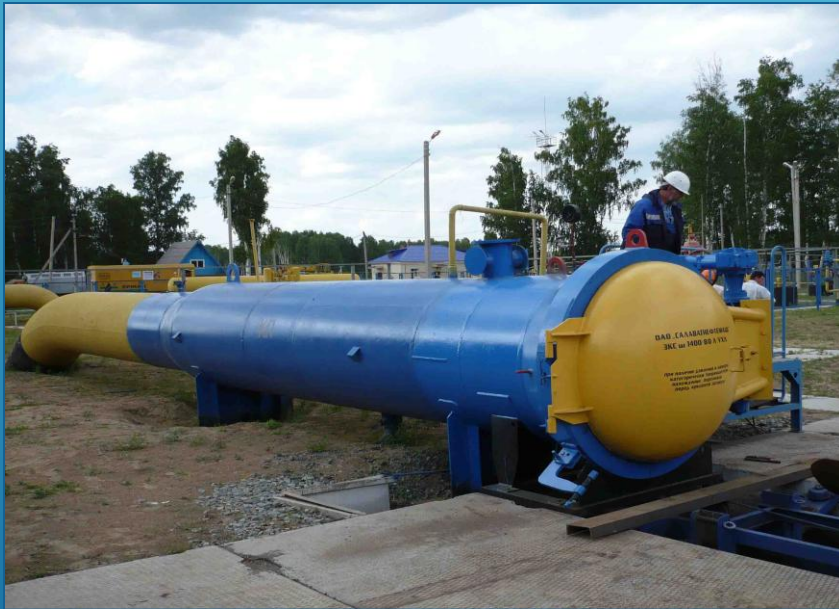
Sector end gate at cleaning and diagnostics devices launching/receiving chamber
