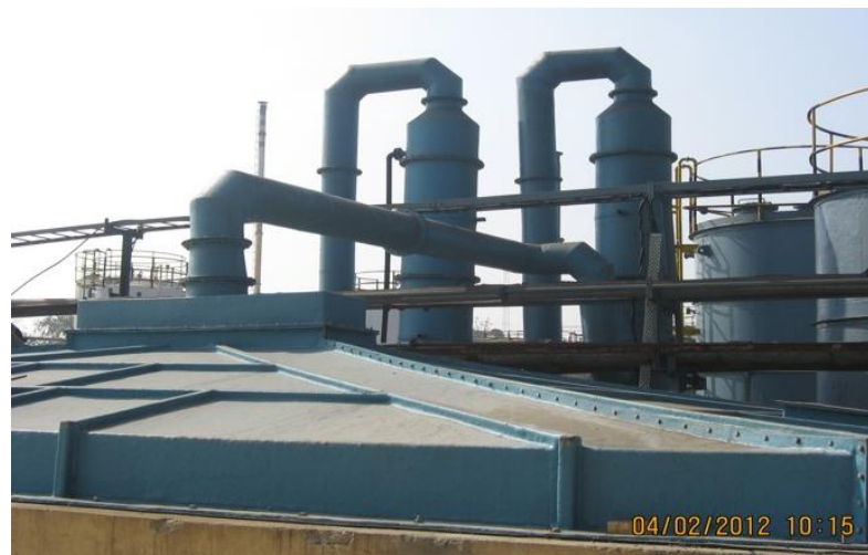
Hood System with Scrubber for Effluent Storage tanks
