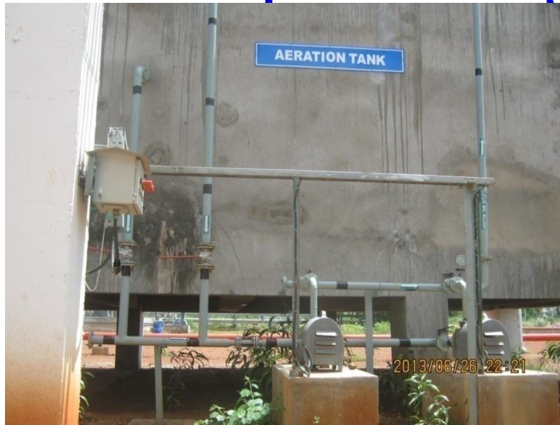
Biological Treatment Plant
